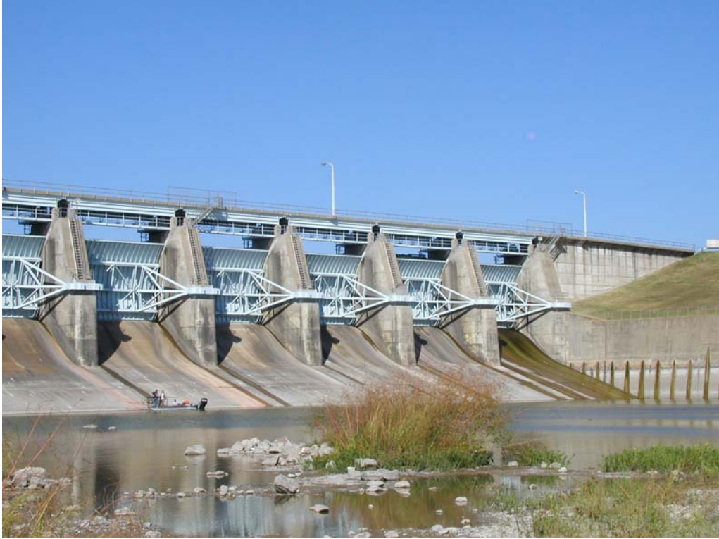
Figure 3-31. Lake Ray Hubbard Stilling Basin
