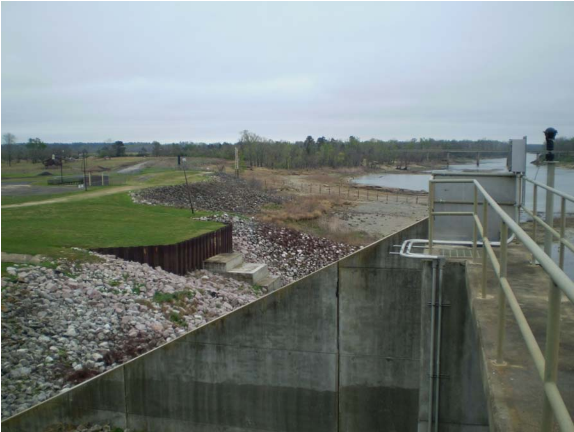
Lake Livingston Dam Tailrace area and east downstream shoreline under low-flow conditions (approx. 1,000 cfs). Photo taken 3/11/09.
