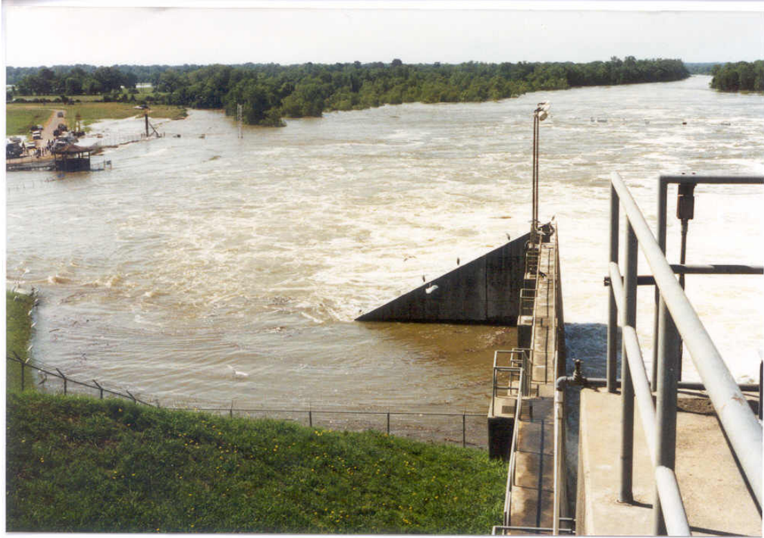
Lake Livingston Dam tailrace area and east downstream shoreline under flood conditions (approx. 90,000-100,000 cfs). Photo taken May 1990.
